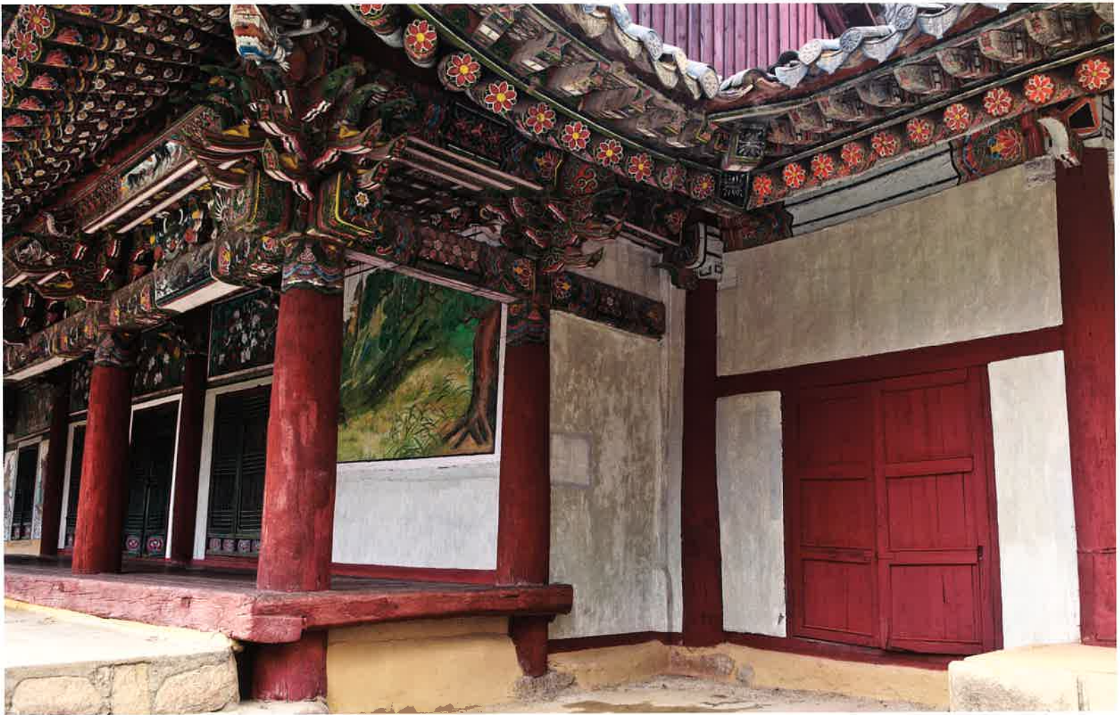
관음전과 동쪽 날개채 연결구조 / 觀音殿·西側 翼舍 結構 / connecting structure between Kwanŭmjŏn hall and eastern wing building
