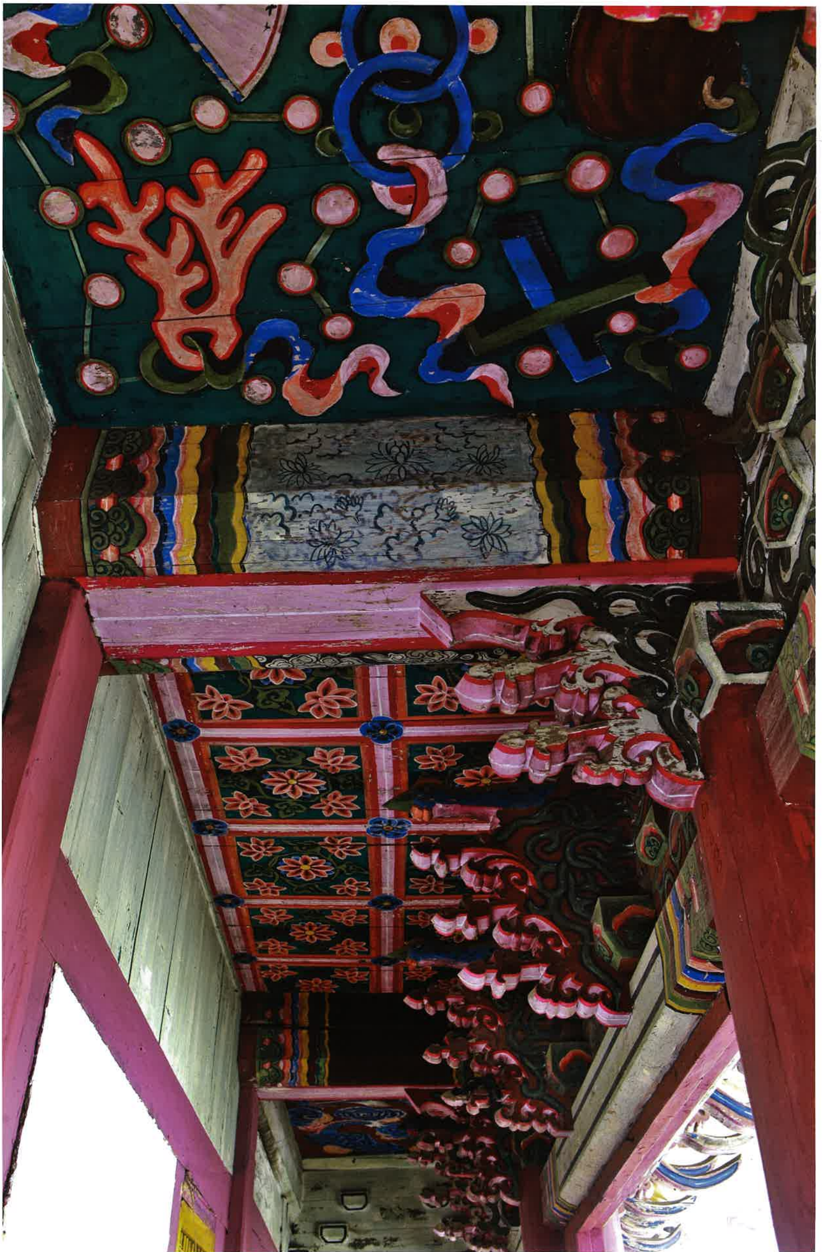
능인암 뒷간 반자 / 能仁庵 退間 天障 / ceiling of space with extra poles outside the inner fence, Nünginam
