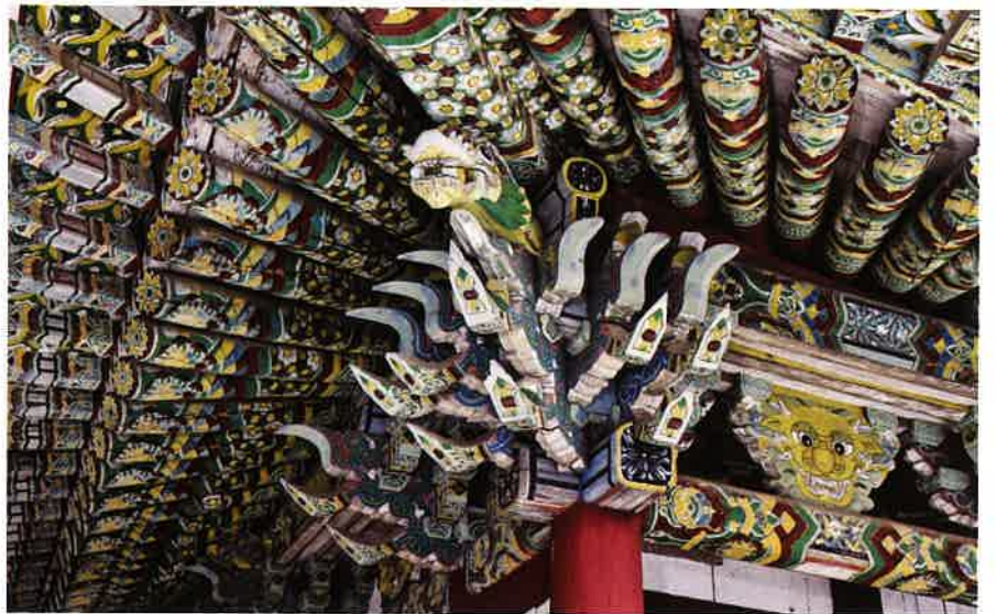
불영암 앞면 서쪽 귀포 / 佛影庵 前面 西側 耳包 front western corner brackets, Puryongam
