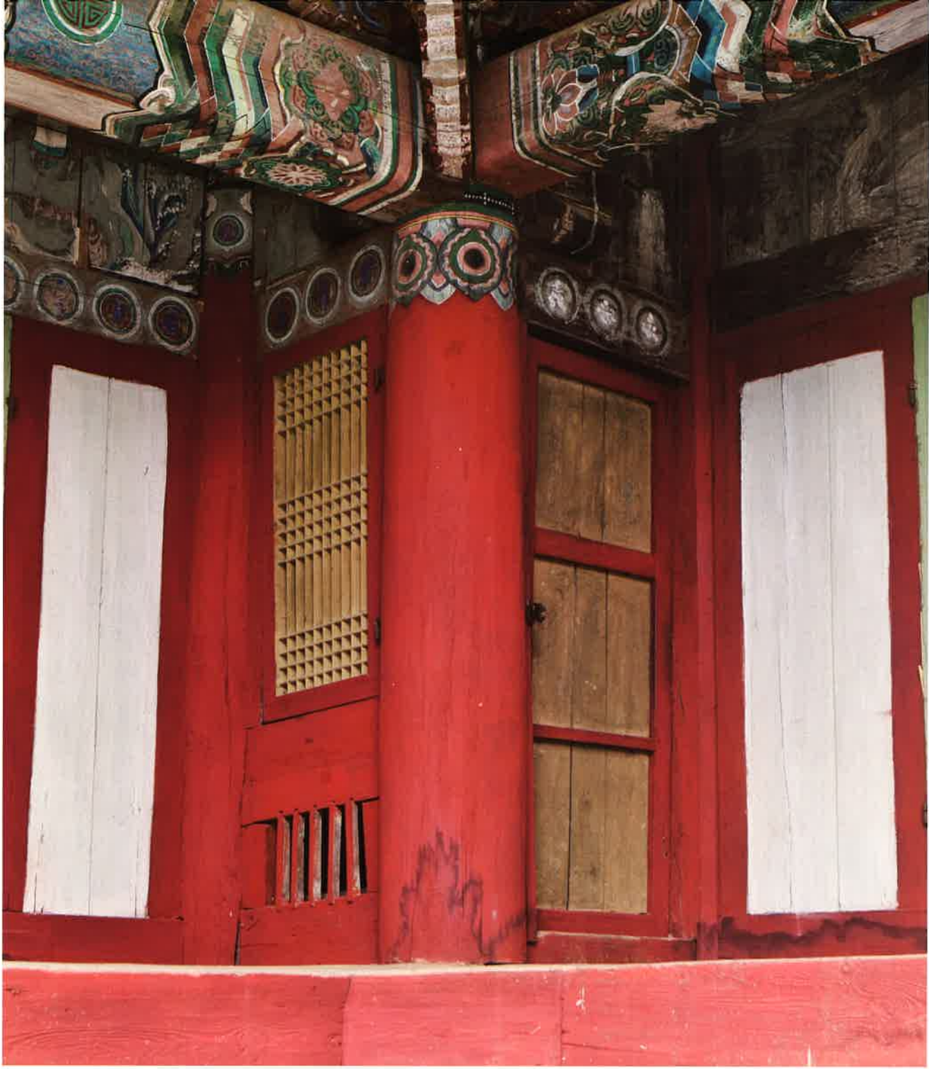
축성전 기본채와 동쪽 날개채 연결구조 / 祝聖殿 基本槩·東側 翼舍 結構 / connecting structure between main building and eastern wing building, Ch'uksongjŏn hall
