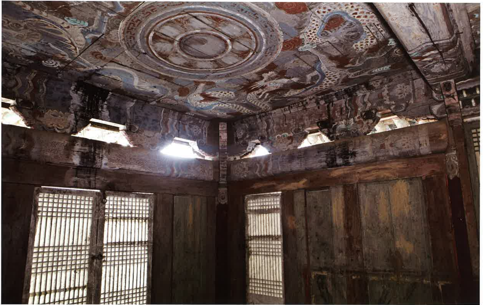
축성전 서쪽 날개채 내부 1 / 祝聖殿 西側 翼舍 內部 1 / inside view 1 of western wing building, Ch'uksongjŏn hall
