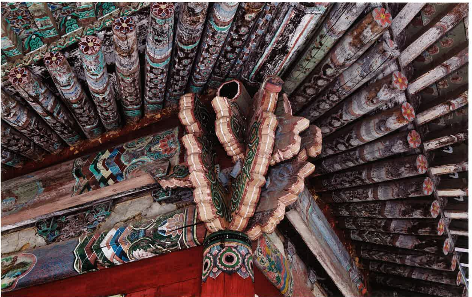
축성전 동쪽 날개채 귀포 / 祝聖殿 東側 翼舍 耳包 / corner brackets of eastern wing building, Ch'uksongjon hall
