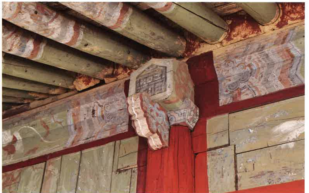
축성전 서쪽 날개채 뒷면 주상포 / 祝聖殿 西側 翼舍 後面 柱上包 brackets above backward columns of western wing building, Ch'uksongjŏn hall
