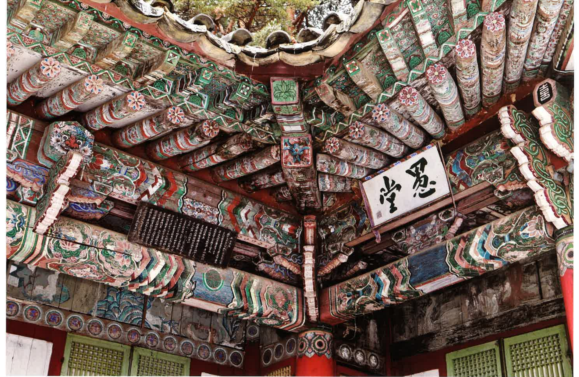
축성전 기본채와 동쪽 날개채 연결구조 / 祝聖殿 基本架·東側 翼舍 結構 connecting structure between main building and eastern wing building, Ch'uksongjŏn hall
