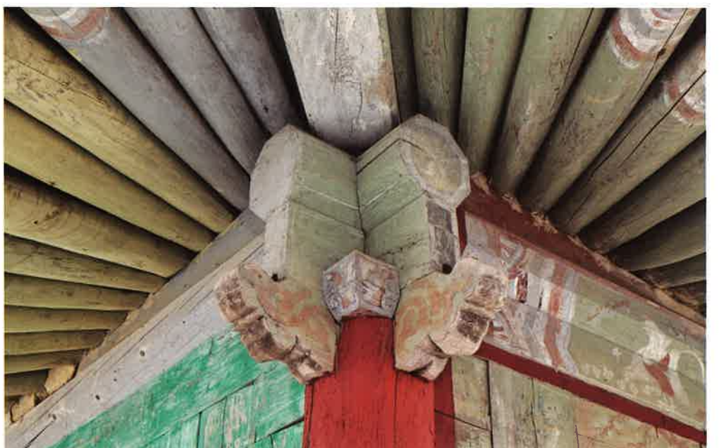
축성전 서쪽 날개채 뒷면 귀포 / 祝聖殿 西側 翼舍 後面 耳包 backward brackets of western wing building, Ch'uksongjŏn hall
