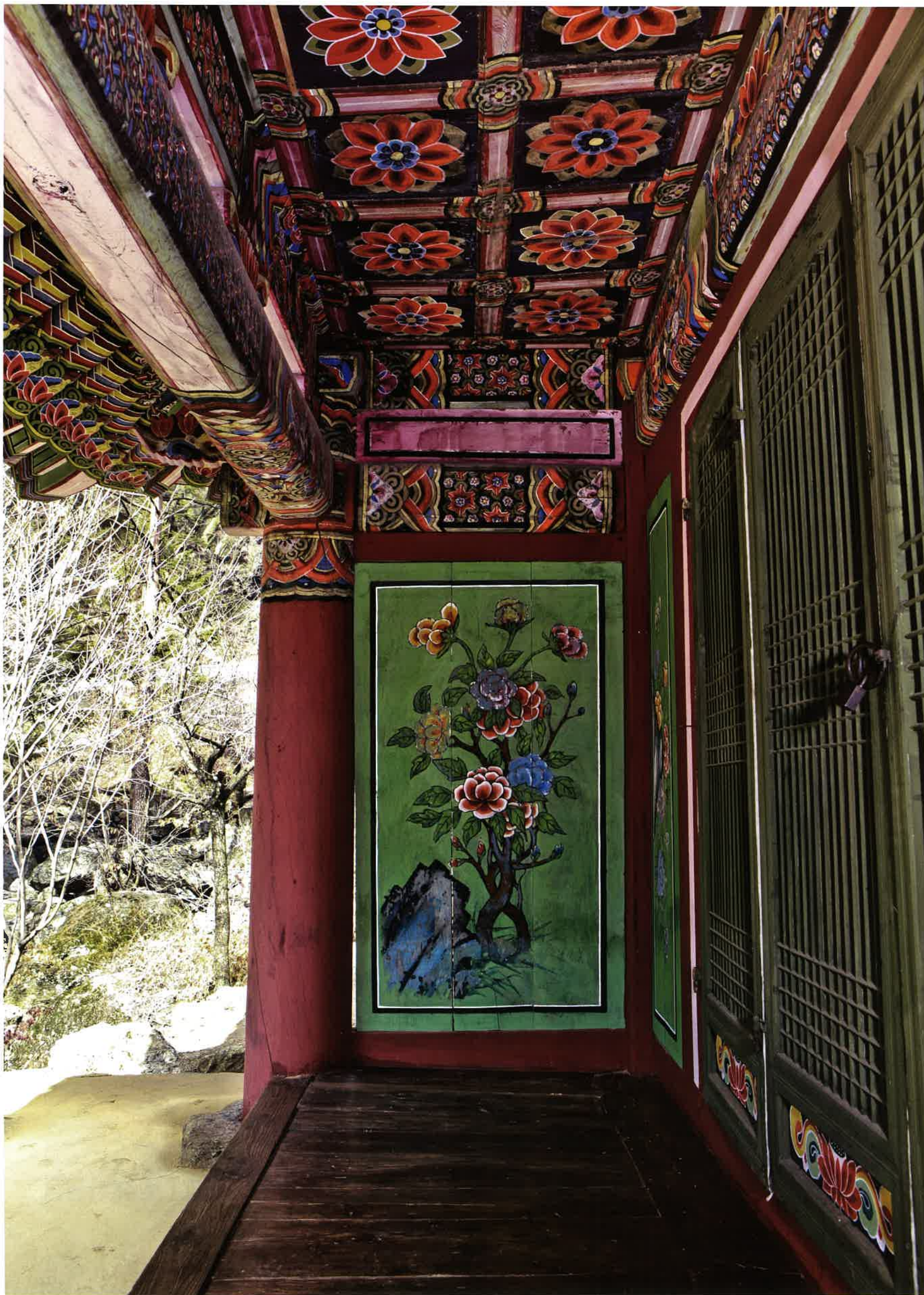
보련대 뒷간 / 寶蓮臺 退間 / space with extra poles outside the inner fence, Poryöndae
