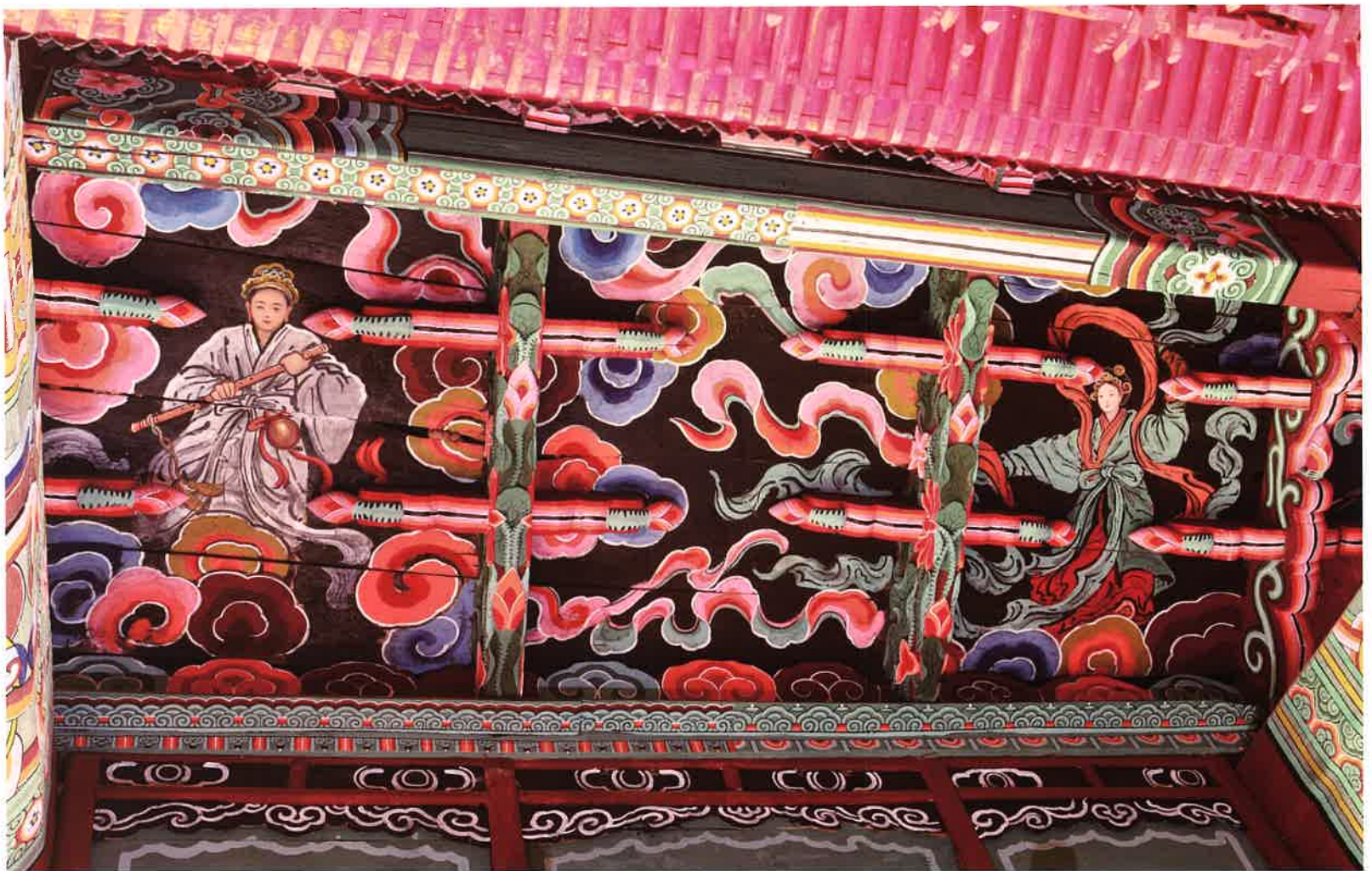
극락전 내부 빗반자 별화 2 / 極樂殿 內部 斜天障 別畫 2 / attached painting 2 on inclined ceiling, Kūngnakchön hall
